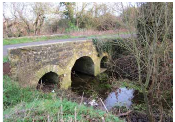
Figure 5: The Grade II Listed Chil Bridge, facing northeast with Thornbury Green houses in the background
