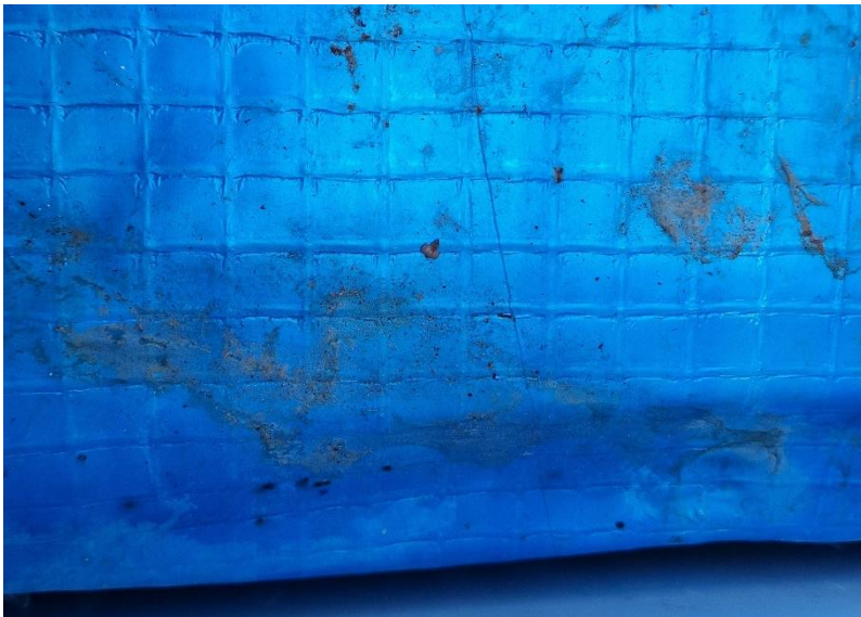
Water staining on VCL
