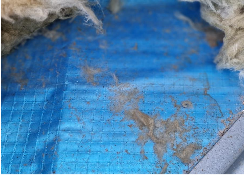
Water staining on VCL surface
