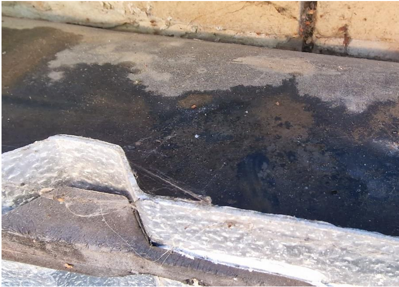
Water was present on top of the cladding rails.
