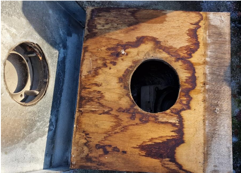
Water staining to plywood support under aluminium vent cap
