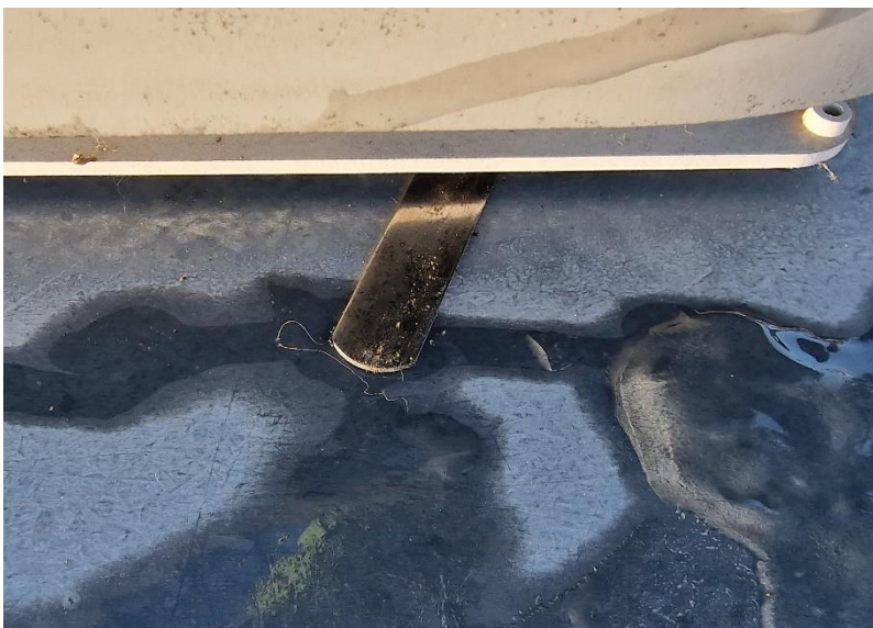
The joint between plastic vent and aluminium vent cap is not effectively sealed
