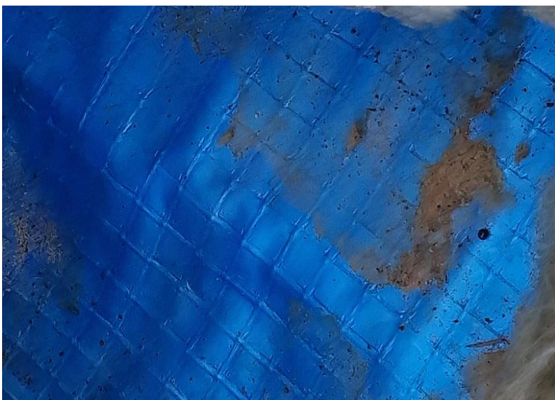
Water staining on VCL
