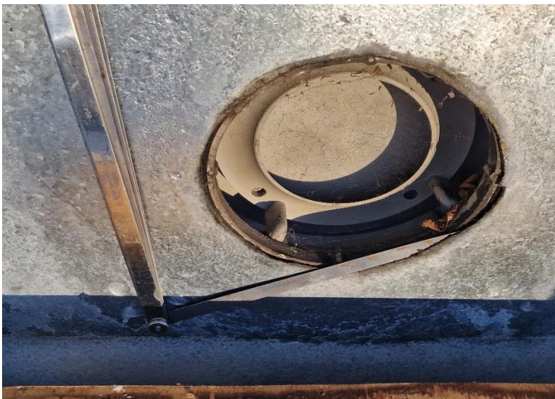
The joint between plastic vent and aluminium vent cap is not effectively sealed
