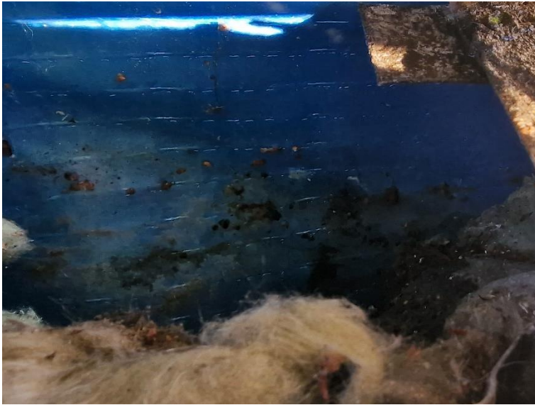
Water staining on VCL where it turns up at the roof lights
