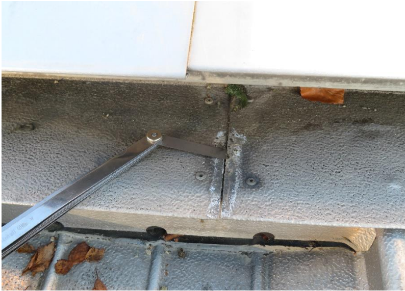
Further evidence of failed but joints in the drip flashings to the roof lights
